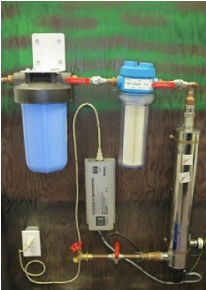
An example of a filter and ultraviolet disinfection system.
