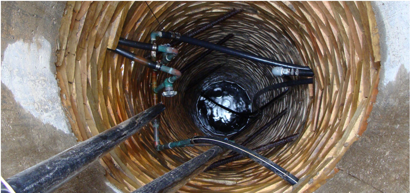
A dug well that is over 100 years old. Moisture seen on the concrete and tile casings indicates that surface water is getting into the well. Ensure that the well is constructed and maintained properly to reduce potential contamination from entering the well.
