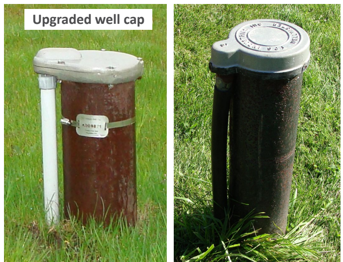
A properly constructed drilled well. The well cap should be upgraded to make the well more secure (pictured at left).
