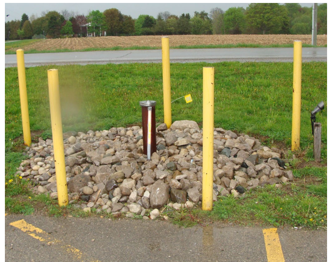
Wells located near the road or parking lots may be at risk of salt (sodium) and vehicle-related contamination. Know what can get into your well and take measures to minimize the potential contamination and the risks.
