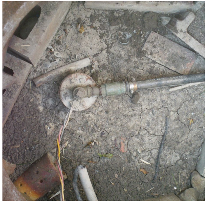
The soil is cracked, evidence that water has entered the well pit (not to be constructed this way anymore) and dried. One way to prevent this from happening is to upgrade the well by installing a pit-less adapter and extending the well casing at least 40 cm above the ground; and ensuring that construction/maintenance is conducted properly. New construction wells cannot be located in well pits. NEVER ENTER A PIT.
