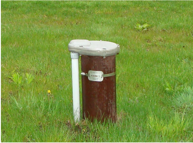
This image shows a properly constructed drilled well with a vented and vermin proof well cap, electrical conduit for submerged pump (to left of well casing), identification tag (linked to Water Well Record), casing extends at least 40 cm above the ground, and ground around the well that is sloped away from well casing to help direct water away from the well.
