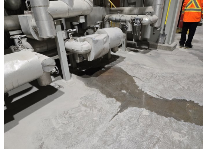
Photo 30: View of a water leak in the Boiler Building.
