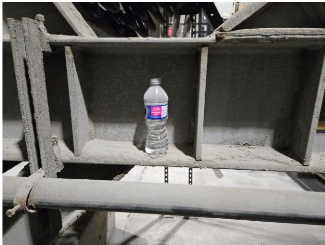
Photo 31: View of plastic water bottle in the Boiler Building.
