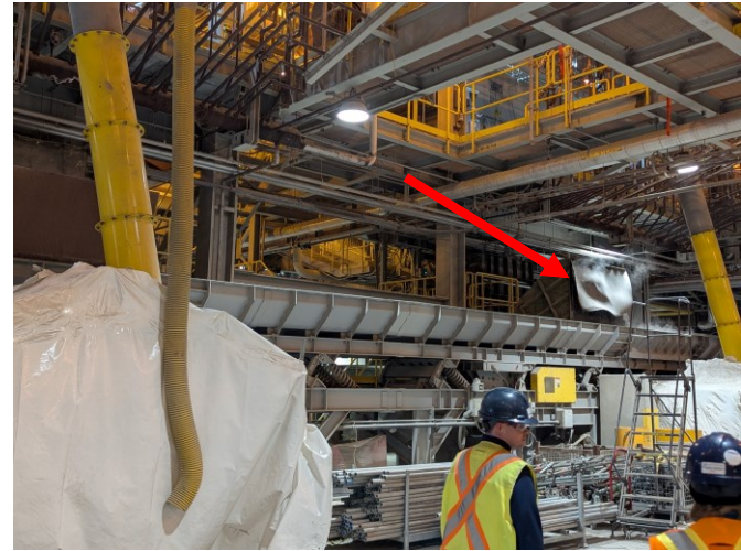
Photo 18: View of operational ash chute cover/baffle.
