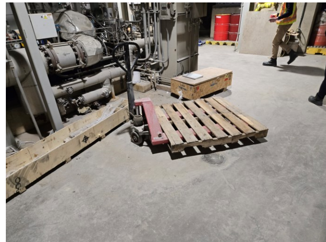
Photo 16: View of wooden skid within the Boiler Building.
