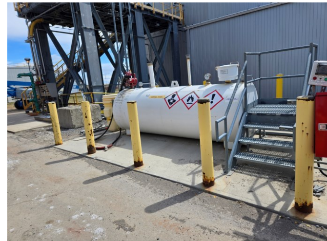
Photo 40: View of the diesel storage tank, north of the Residue Building.
