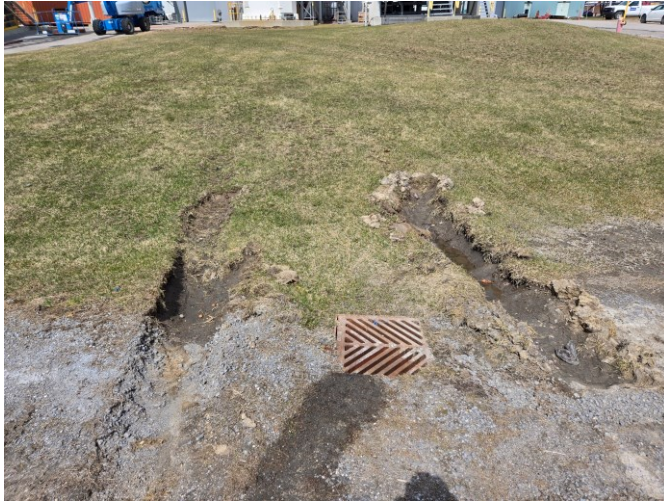
Photo 21: View of ruts near the ammonia storage tank.
