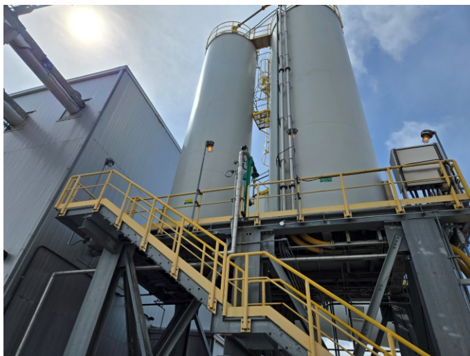
Photo 35: View of Pozzalon and Cement Silos.
